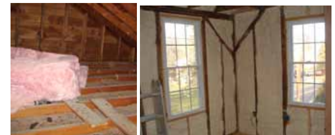
Figure 9.1: There are a number of techniques to improve the energy efficiency of existing buildings without destroying the appearance of it: Internal wall and loft insulation.
